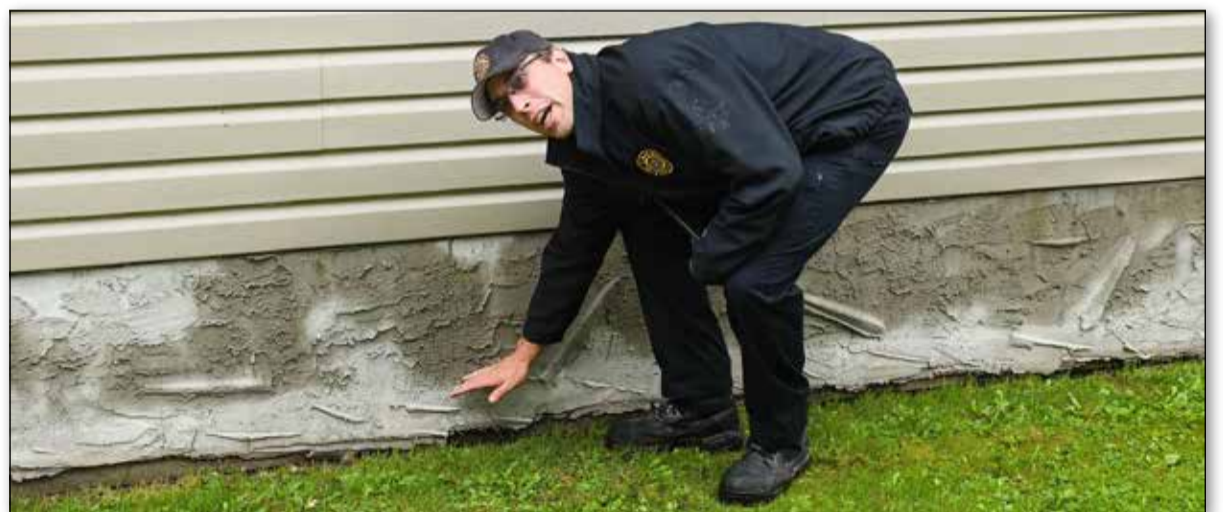
Firefighter Terrance Corke highlighting a space between the stucco and wood.
