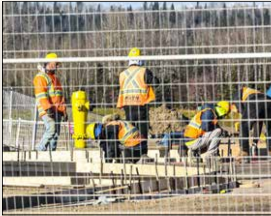
Construction of the new roadway at Festival Park is nearing completion. Crews have paved the traffic circle connecting the old entrance/exit to a new entrance/exit near the Seniors Circle. Anticipation is high for the fence to come down and for drivers to get their first taste of the updated roadway. On Saturday, a construction worker crew was seen through the fence working on the curbs in front of the Seniors Circle.
