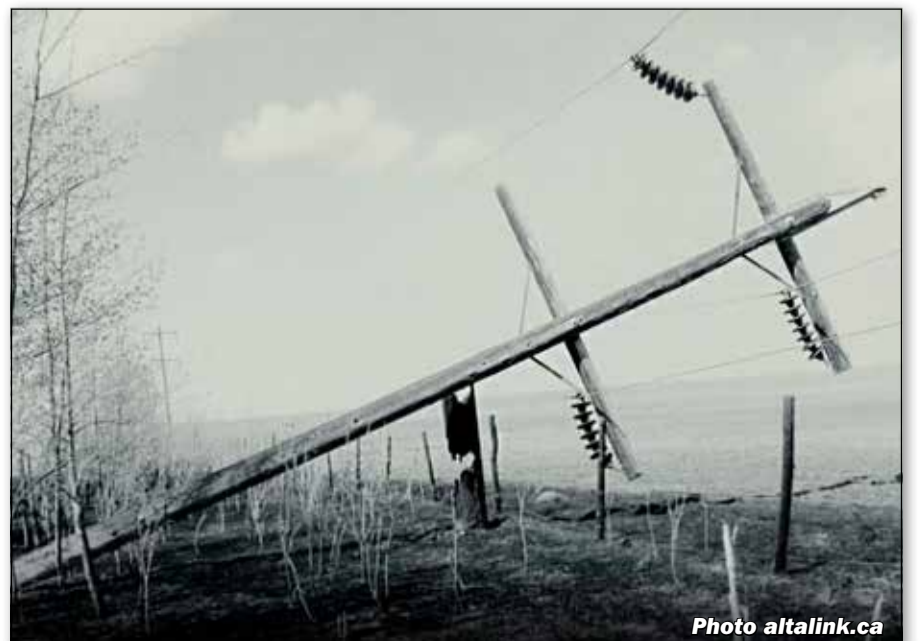
A damaged power pole.
