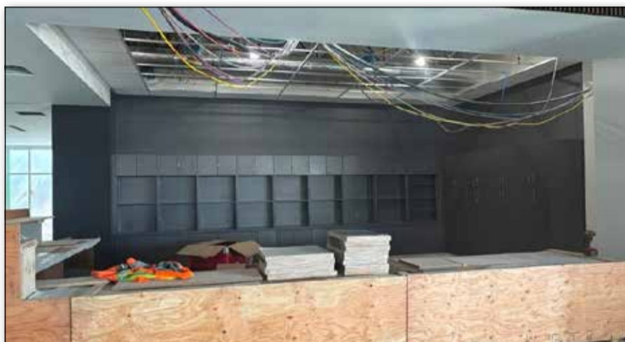
Construction of the Canfor Culture & Events Centre is now 89 per cent complete and remains both on budget and on schedule. Interior and exterior finishing work is currently underway, with flooring being installed. Landscaping is also expected to begin this month. The facility has been designed with community use in mind, featuring a range of purposeful spaces intended to support connection and learning. It includes gathering areas to encourage community engagement, as well as gallery spaces for art exhibitions. The theatre within the centre is planned to accommodate a wide variety of programming, including performances, events, conferences, festivals, and ceremonies.
